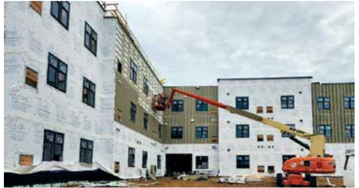
Workers used a crane to install siding on the main building last September.
