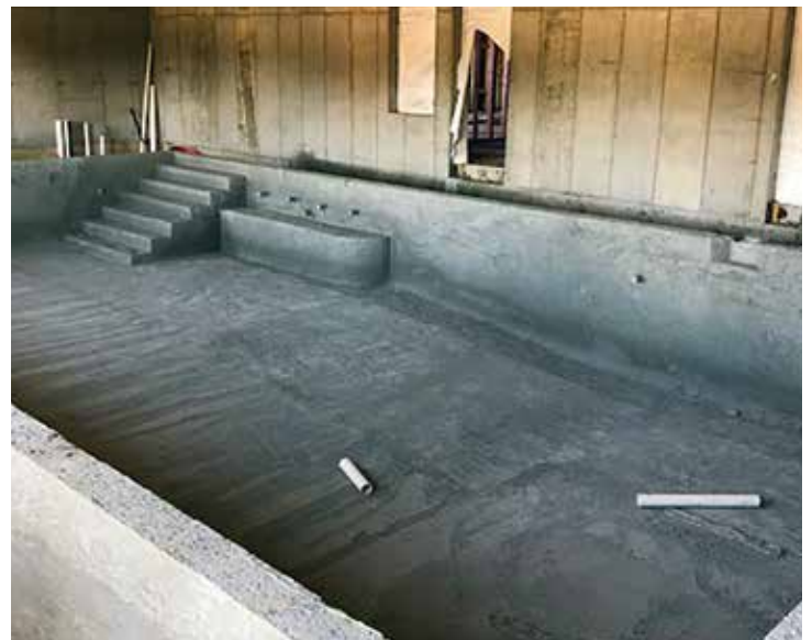
By August 2022, progress had been made on what will likely become one of the most sought-after amenities on campus: a warm water pool.
