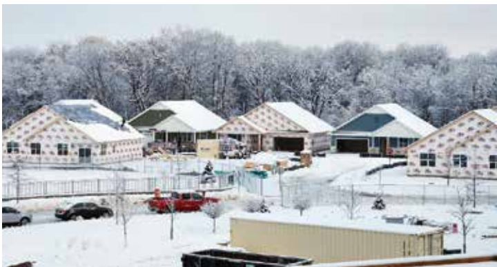
Taken in December 2022, this photo shows five of the 20 detached rental townhomes that are being constructed on the north end of campus.
